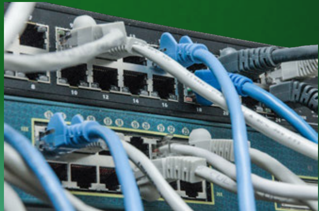
Ethernet cables plugged in to Ethernet switches in a server room. Photo by Jon 'ShakataGaNaI' Davis, Wikimedia Commons
